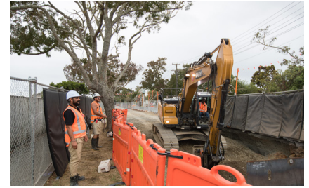
Trenching at a Piritahi site in Hendon Avenue, Ōwairaka, to upgrade the existing stormwater and wastewater systems
